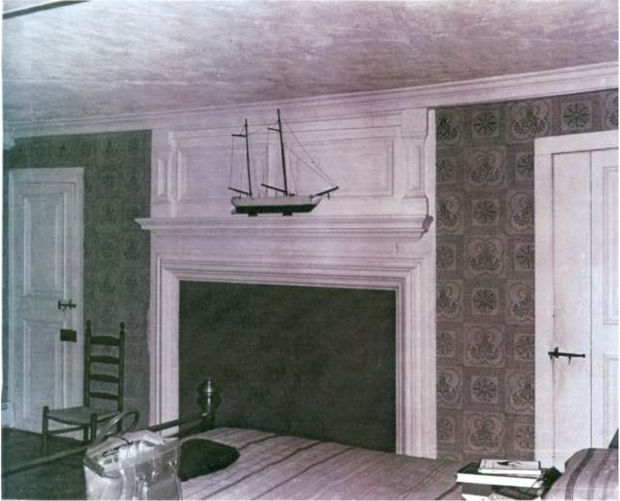
Fireplace wall of north-west room (Lafayette bedchamber) on second floor, with paint of 1950's applied over original marbled trim, which is to undergo restoration. Photograph: Robert H. Zexter and Nancy Zexter, 1971
