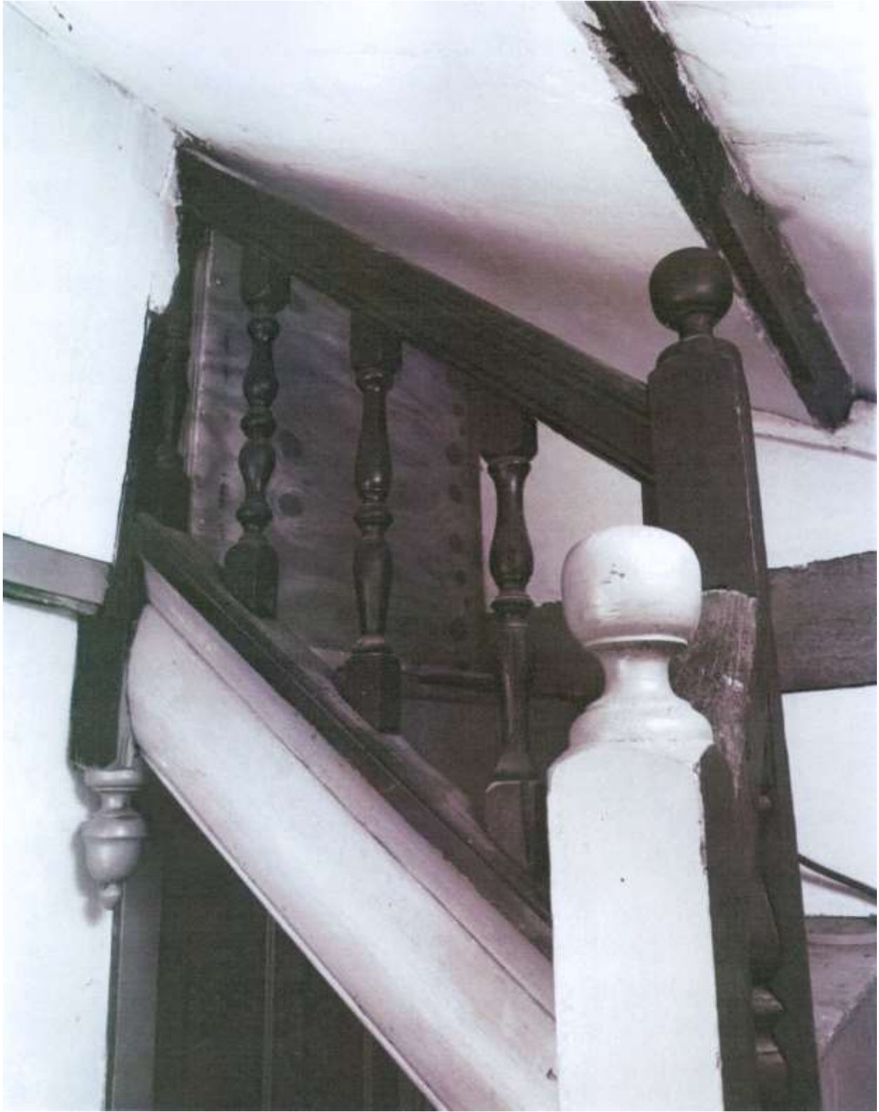
Fully finished stairway from third floor into garret, showing rafters of roof at banister height, Photographer: John Shotwell, 1982
